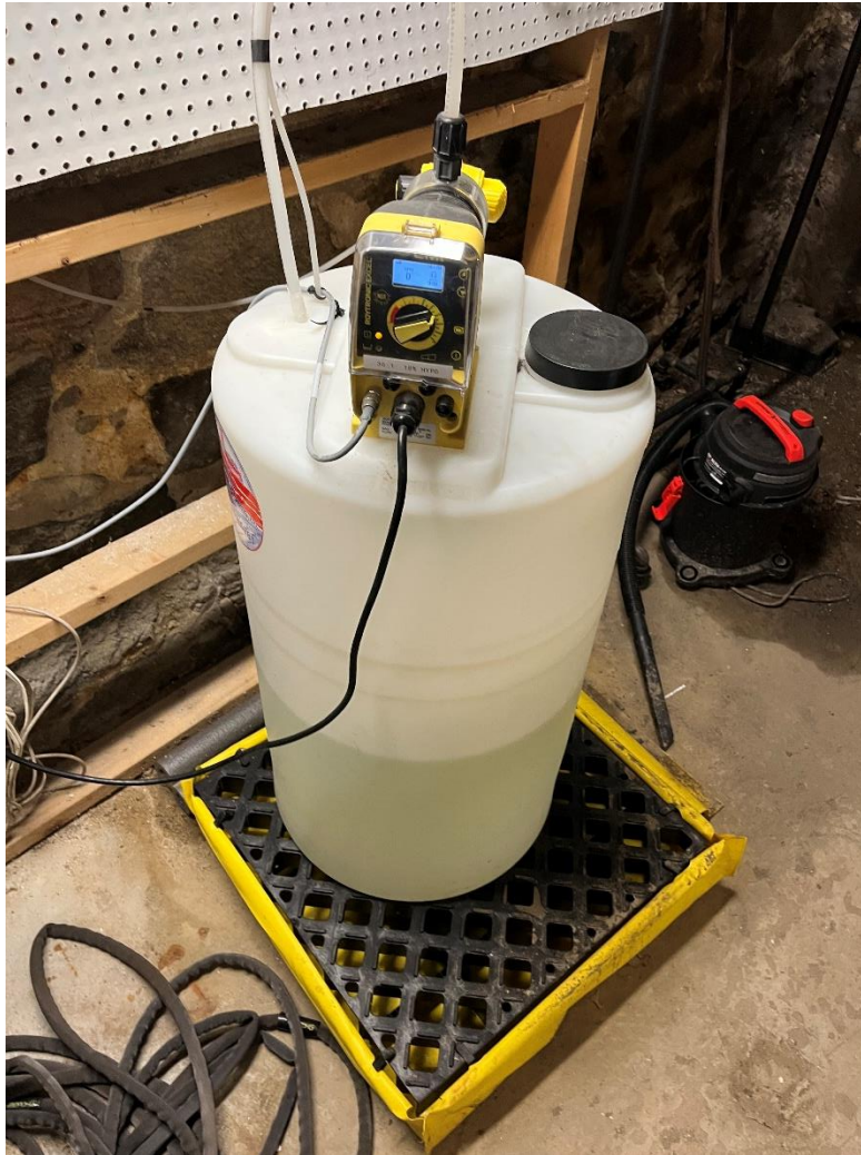
Hypochlorite Storage Tank
